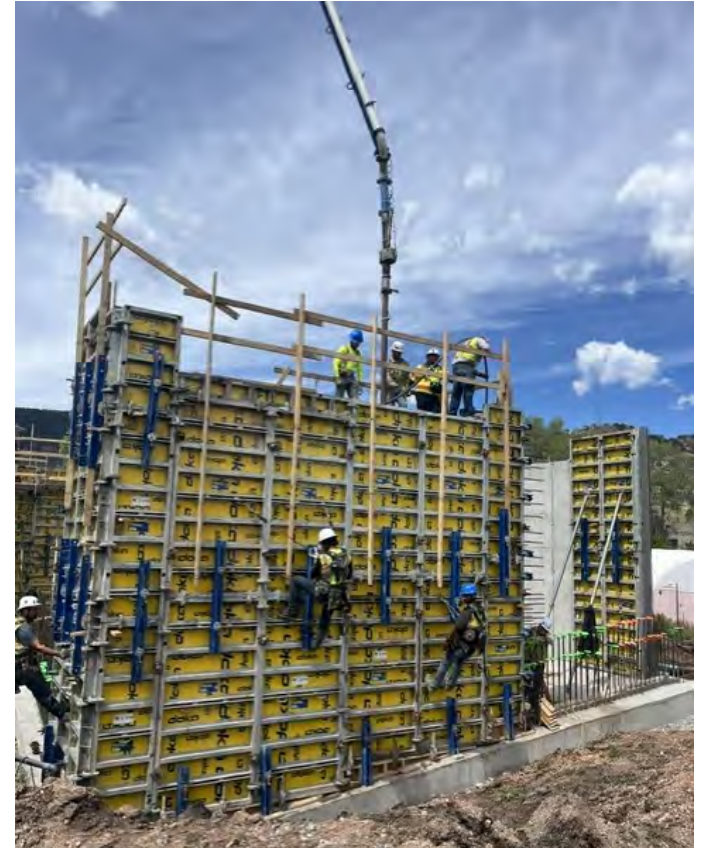
PERRY PARK WWTF
