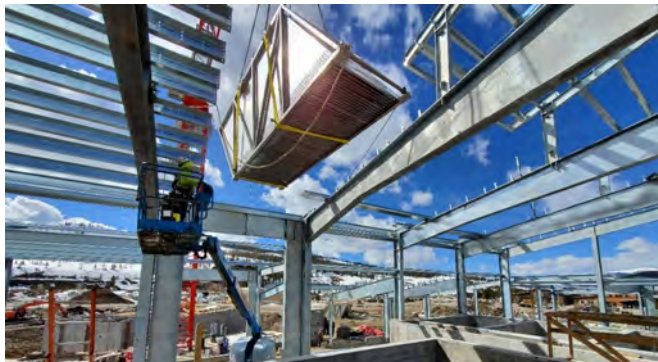
Breckenridge 2 nd Water Treatment Plant
