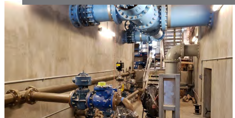
BRECKENRIDGE 2 ND WTP
