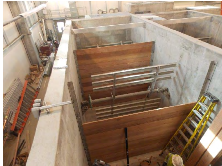
Breckenridge 2 nd WTP
