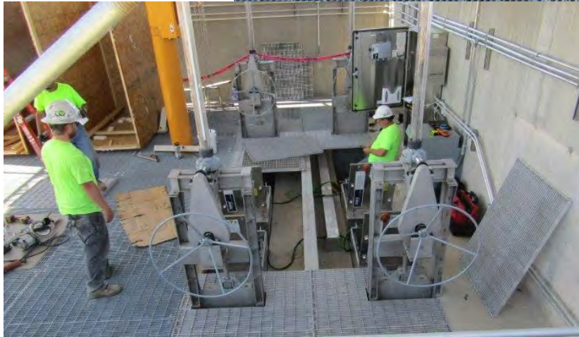
SECURITY WWTF IMP.
