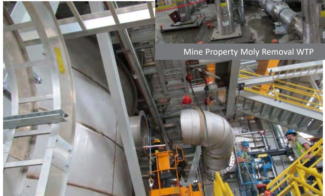
Mine Property Moly Removal WTP
