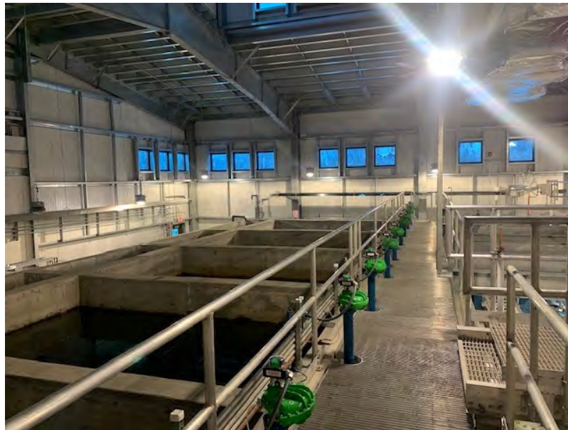
Breckenridge 2 nd Water Treatment Plant
