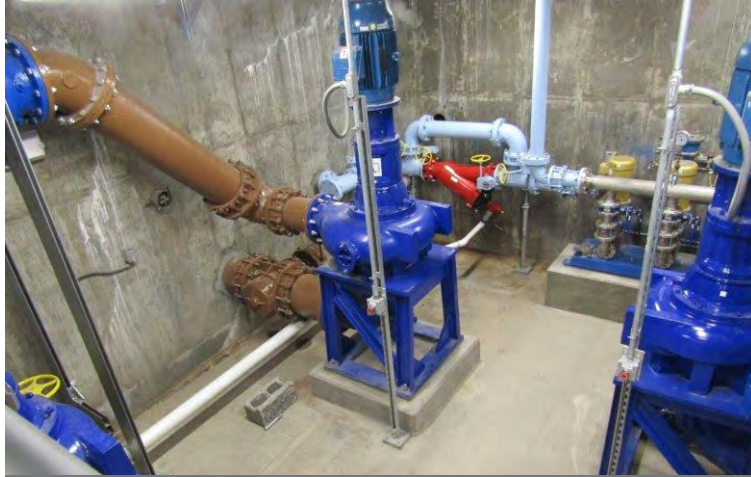
SECURITY WWTF IMP.
