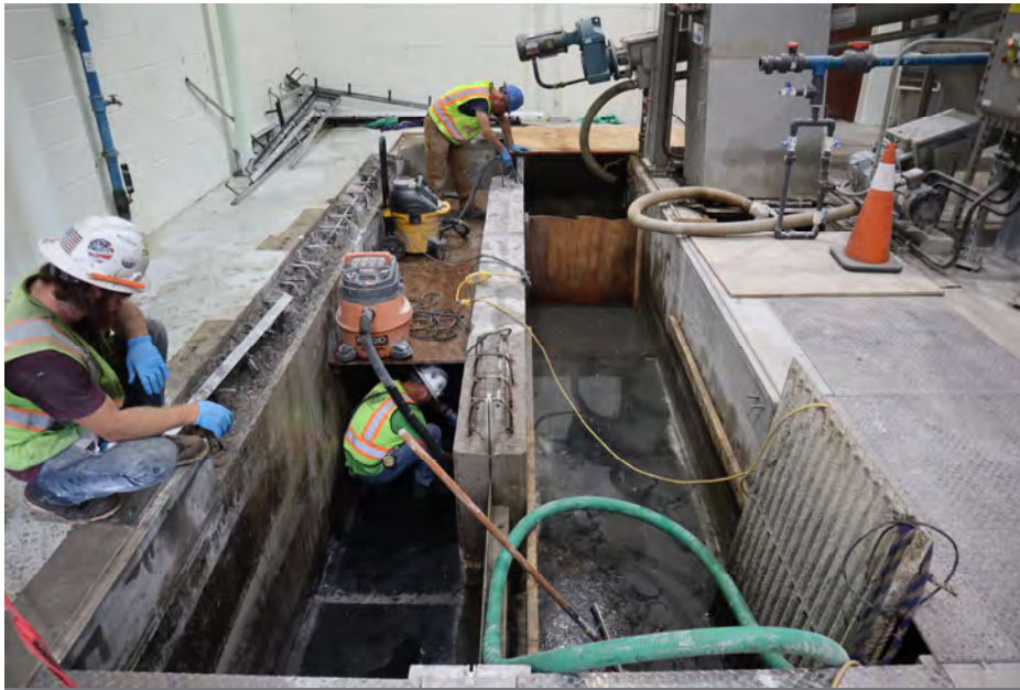
Avon WWTF Nutrient Upgrades
