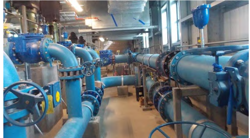
BRECKENRIDGE 2 ND WTP – WATER PS
