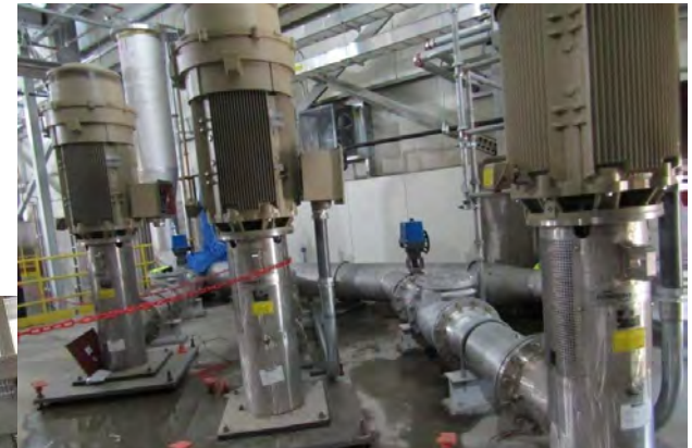
Mine Property Moly Removal WTP
